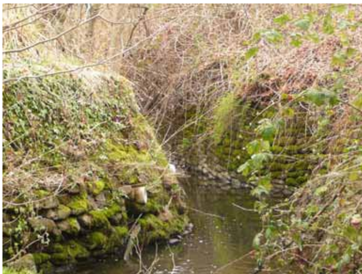
Photos (provided) of channelization and erosion on Bowker Creek.
