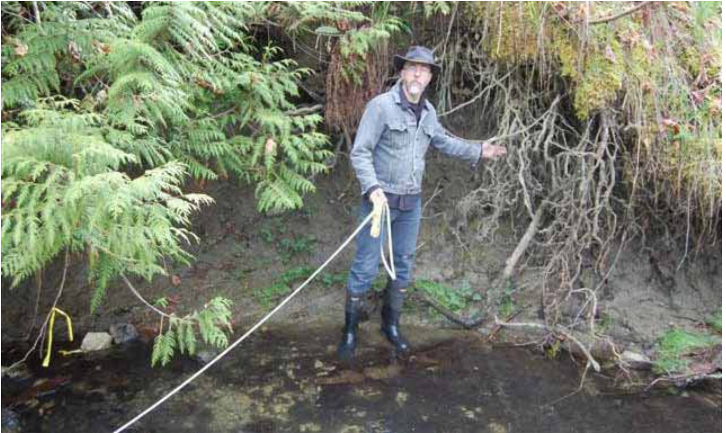
Photo: Stormwater erosion at Douglas Creek. Friends of Mount Douglas Park Society website: http://www.mountdouglaspark.ca/PhotoAlbums/Douglas%20Creek%20Storm%20Surge%20Erosion/index.html?delay=2&fullscreen=yes
