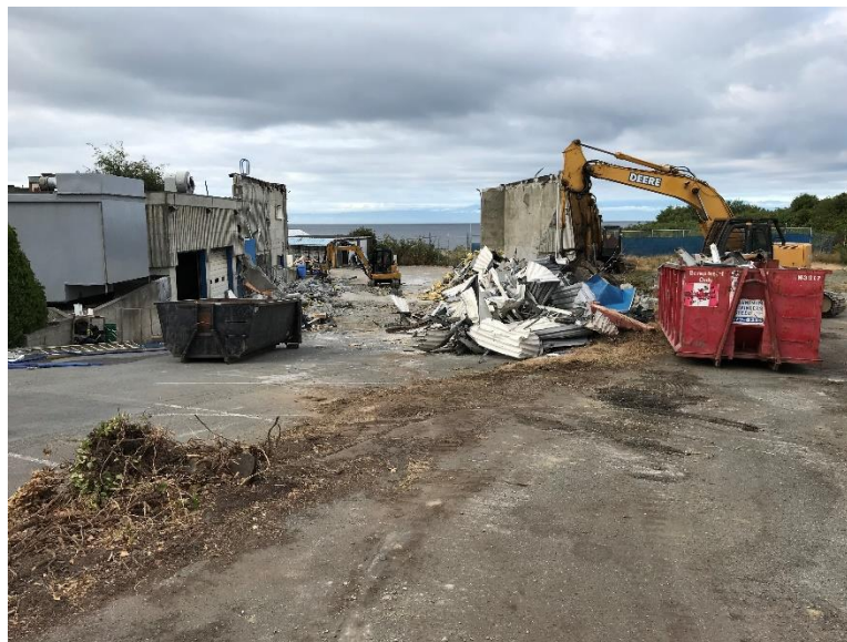
Figure 20 – Demolition of exterior concrete walls and metal roof, sorting material for salvage.
