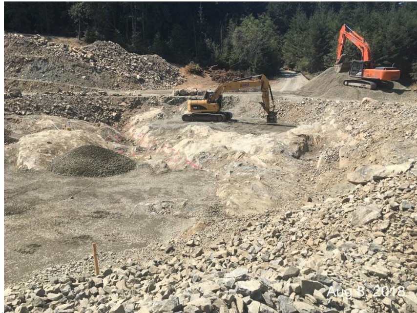
Figure 11 – Excavator with hoe-pack compacting placed aggregate material in valleys and depressions in bedrock.
