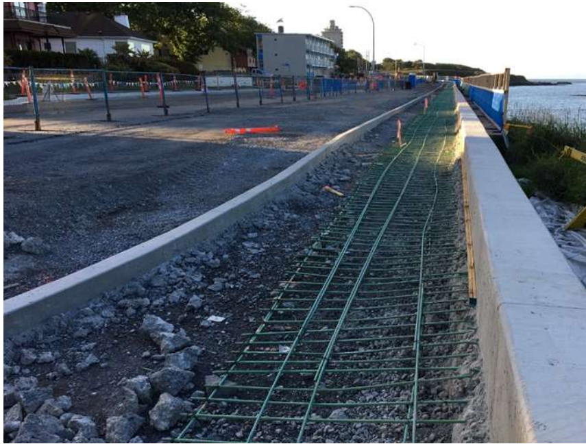
Figure 15–Clover Forcemain- New concrete wall replacing old balustrade wall, rebar installed for sidewalk and concrete curb delineating Cycle Track and sidewalk, Dallas Road from Dock Street looking east.
