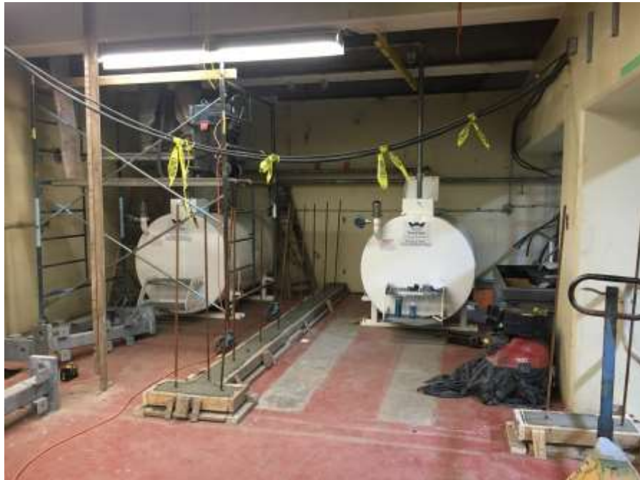
Figure 10–Clover Point Pump Station- Diesel fuel tank storage room location.
