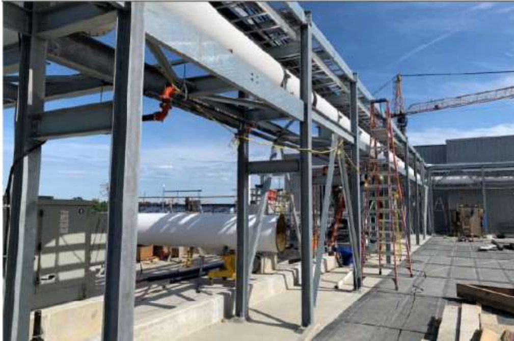
Figure 4- McLoughlin Point Wastewater Treatment Plant- Installation of Hydronic lines to Odour Control roof to unit.
