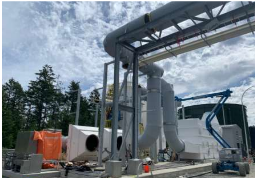
Figure 6- Residuals Treatment Facility- Installation of fiberglass reinforced plastic ducting for odour control systems being installed as well as structural supports.
