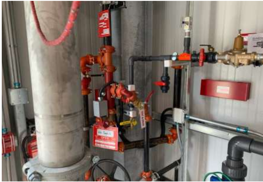
Figure 8- Residuals Treatment Facility – Fire protection water system mechanical installations nearing completion in Water Pump House.
