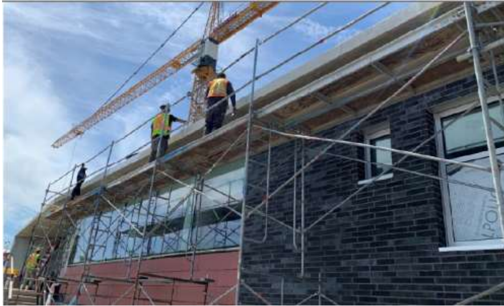
Figure 2– McLoughlin Point Wastewater Treatment Plant - Coating of leading edge Operations & Maintenance roofing.
