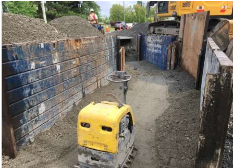
Figure 19–Residual Solids Pump Stations– Marigold Road – Backfilling and compaction of pipe installed on east side of Colquitz Creek.
