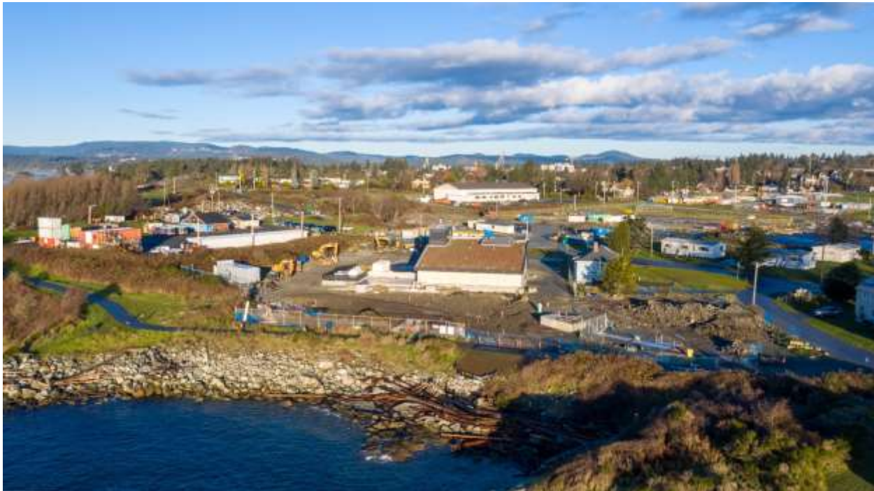
Figure 10 – Looking north towards the Macaulay Point Pump Station (construction in progress, landscaping still to be completed)
