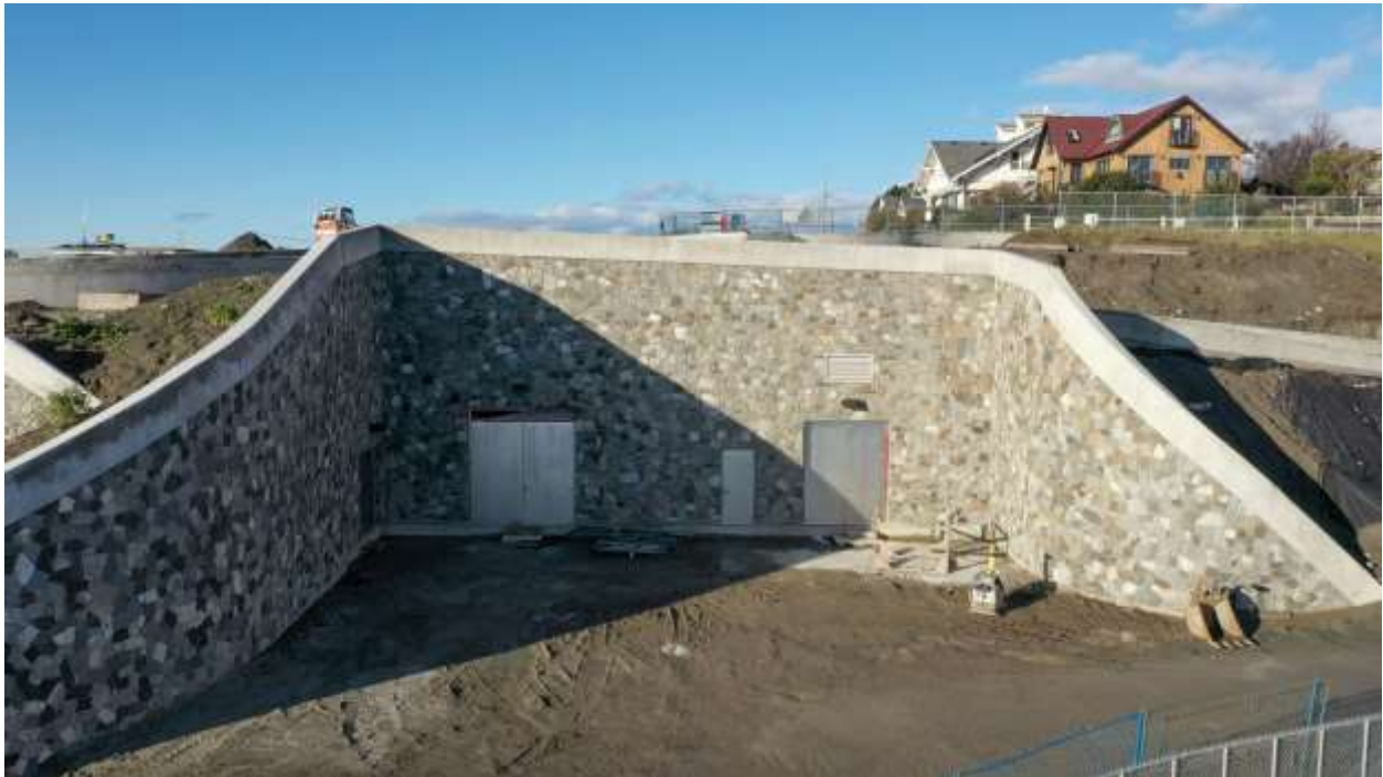
Figure 6 – Entrance to the expanded Clover Point Pump Station (construction in progress: public amenities and landscaping still to be completed)
