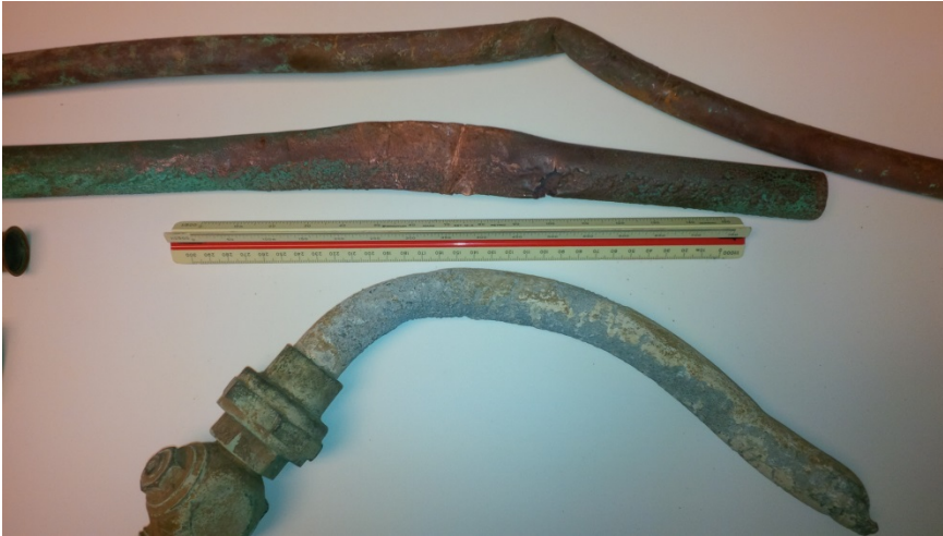
Photo 1- Copper pipe with pin-holes and corroding galvanized metal pipe
