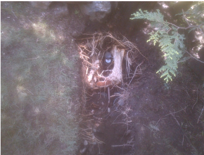
Photo 4 – Water Service Box surrounded by tree roots
