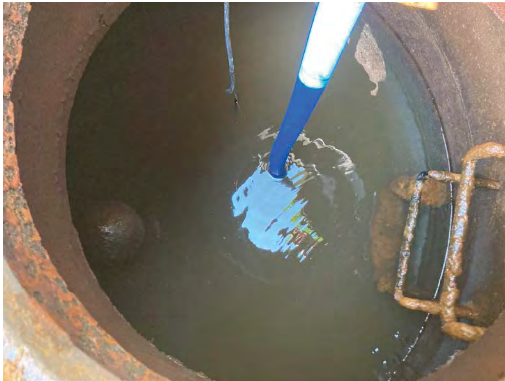
Photo 17: Interior of MH1 after partial lowering of water level using pump. (2022-08-31, JDM)
