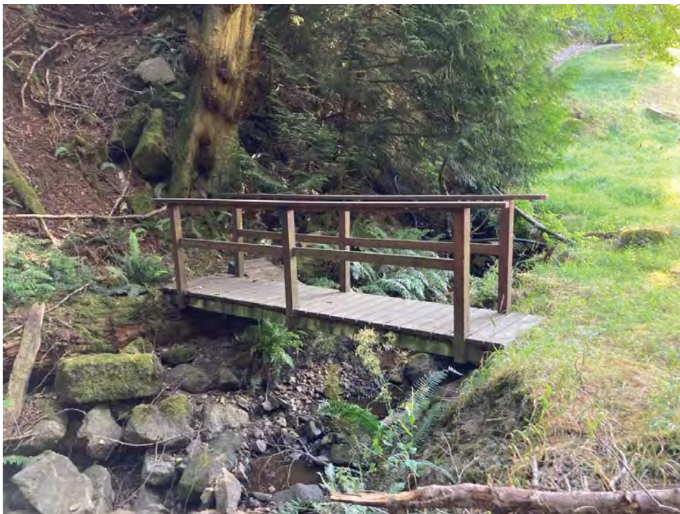
Photo 16: Pedestrian bridge downstream of spillway. Limited armour protection. (2022-08-31, JDM).
