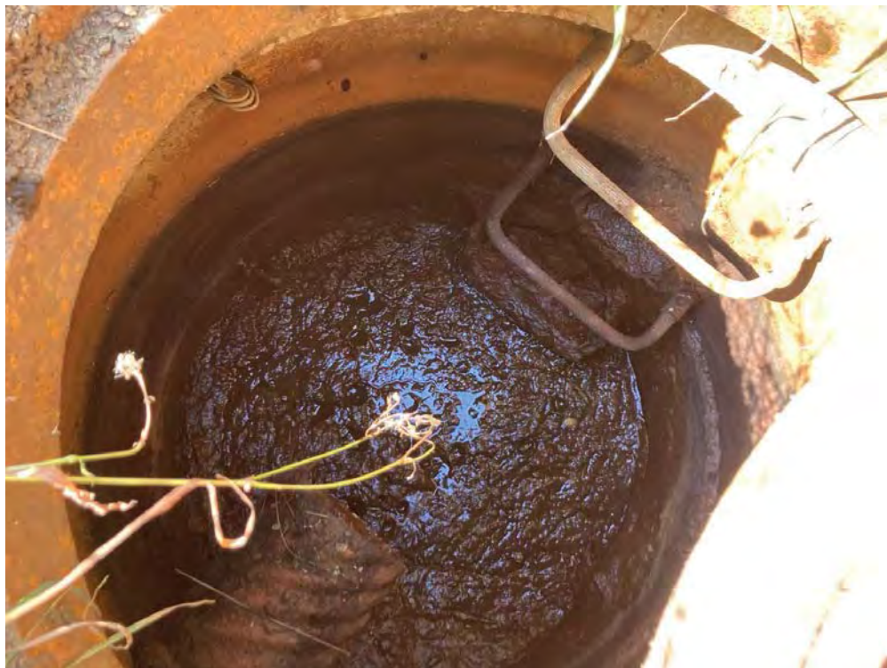
Photo 18: Interior of MH2 – approximately 250 mm of fine sediment. (2022-08-31, JDM).
