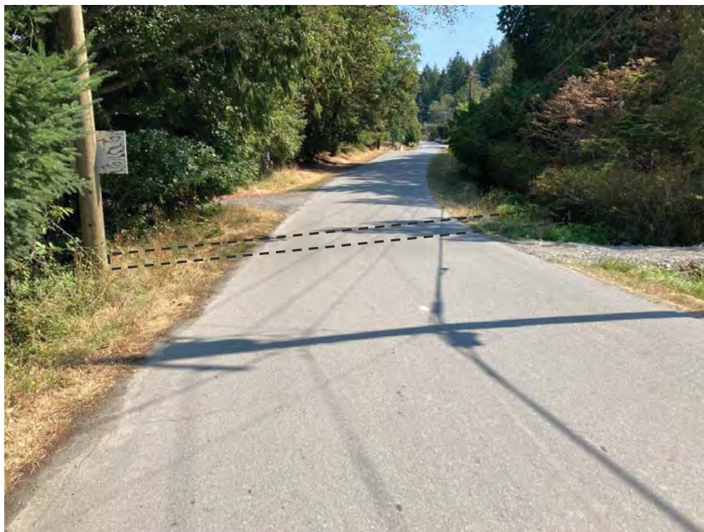
Photo 24: Culvert location on East Point Road ~200 m west of Harris Road. (2022-08-31, JDM).
