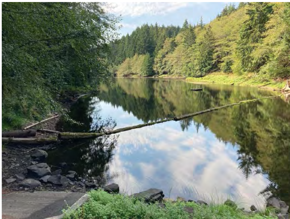
Photo 4: Looking southwest from dam crest at log boom. Intake raft in distance. (2022-08-31, JDM)
