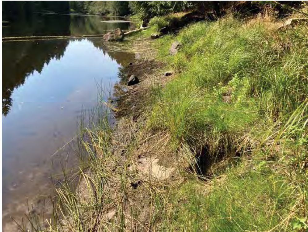
Photo 5: Sinkhole/depression upstream of left abutment. (2022-08-31, JDM).
