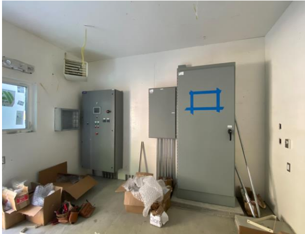
Electrical Room Panels
