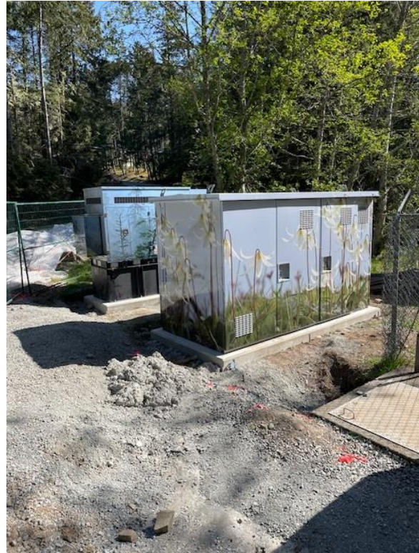
Galleon PS – Kiosk and Genset
