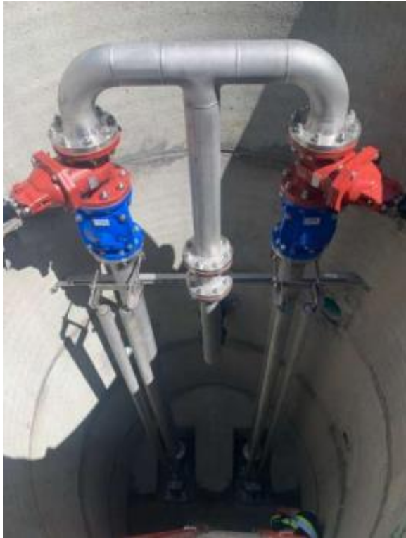
Cannon PS – Pumps and Piping
