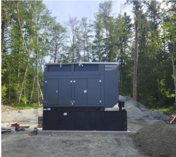
Schooner WWTP Genset
