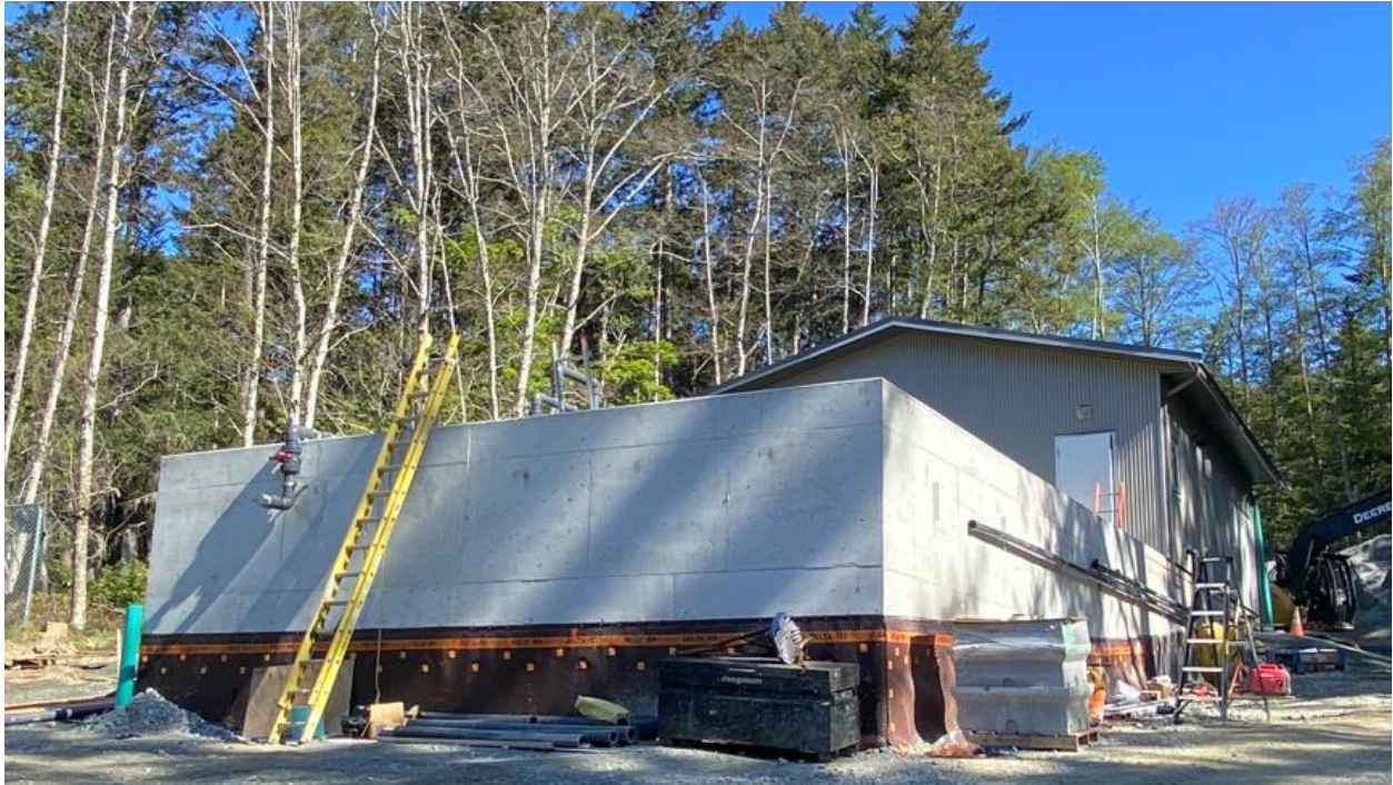
Schooner WWTP Tanks and Operations Building in Background
