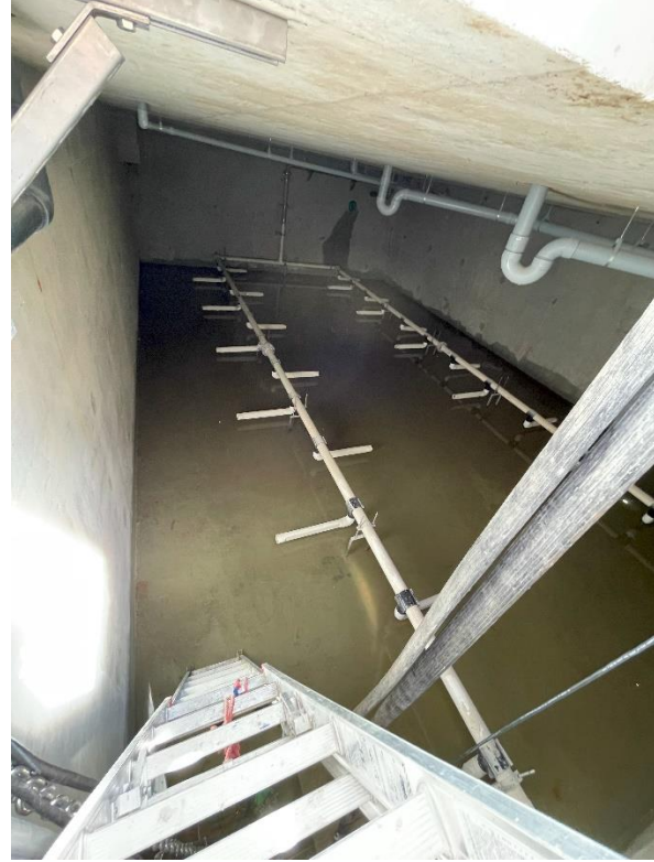
Equalization Tank and Diffusers
