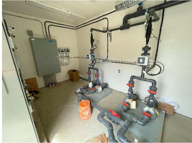
Permeate Pump Room
