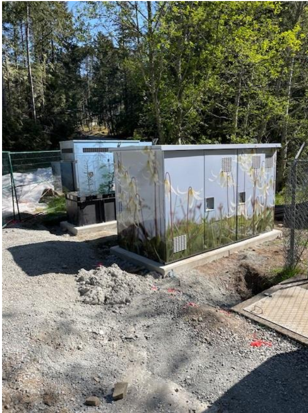
Galleon PS – Kiosk and Genset
