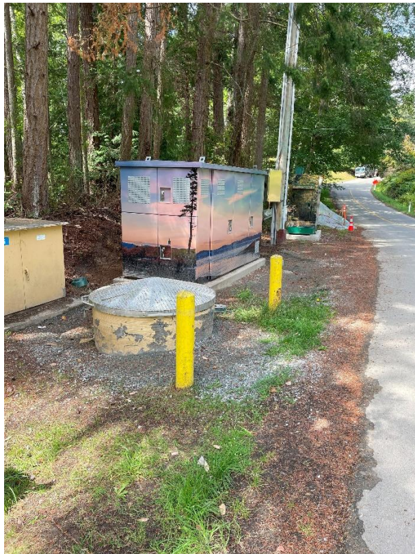
Schooner PS – Kiosk and Genset
