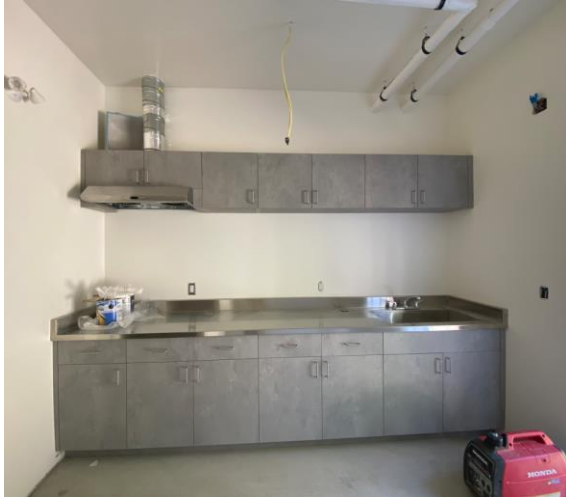
Lab and Control Room
