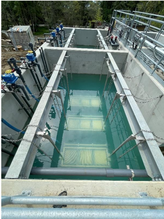
Membrane Tanks and Membranes
