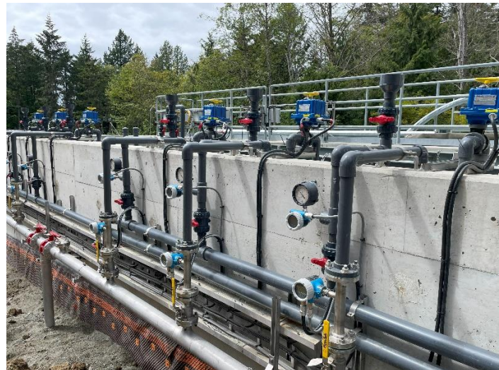
Permeate and Air Piping
