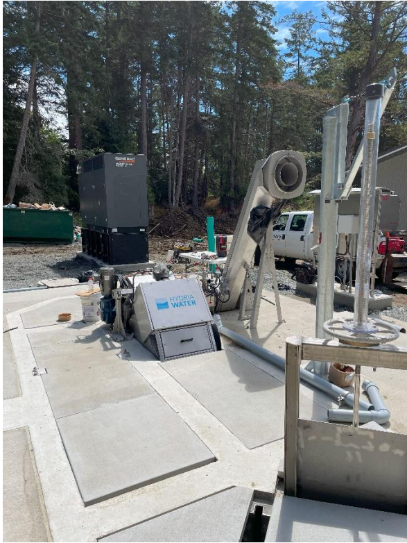
WWTP Screen and Genset
