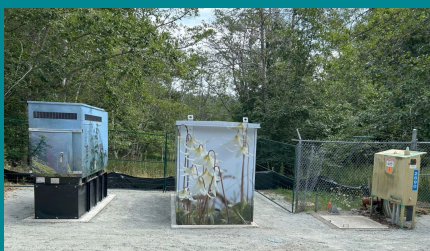
Galleon Pump Station
