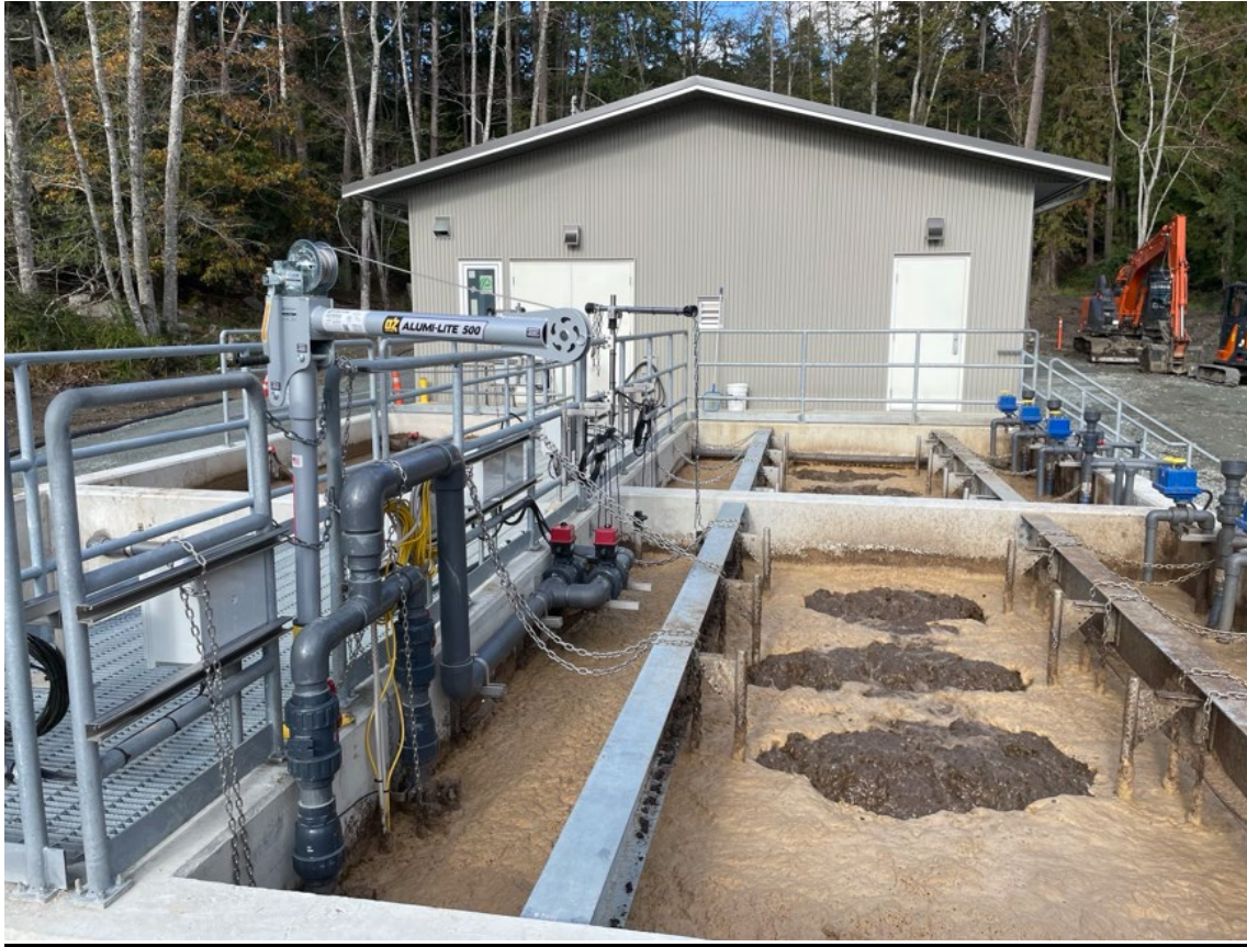
Schooner WWTP in Operation
