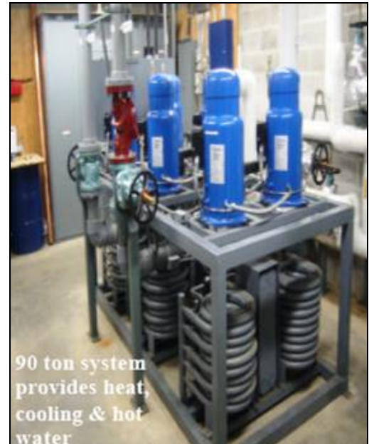
Figure 12: Heat Pump at Pacific Sands Resort, Parksville
