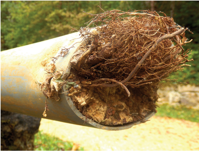
Tree roots entering through cracks or gaps in pipes
