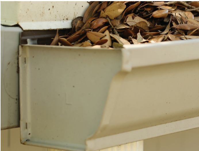
Debris from gutters or cleanouts filling pipes
