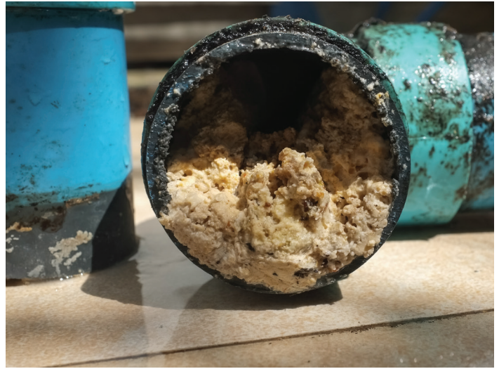
Fats, oils and grease clogging pipes
