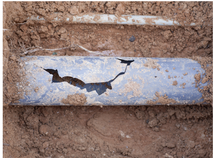
Cracks, breaks, leaks at joints or collapse from shifting ground or deteriorating material
